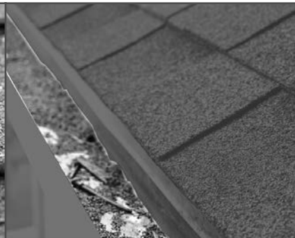
Granules in the gutter indicate shingle deterioration.
